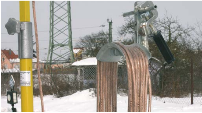
Earthing spike with coiled earthing cable.
