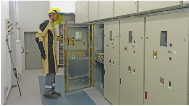
Switch room with insulating mat fitted.
