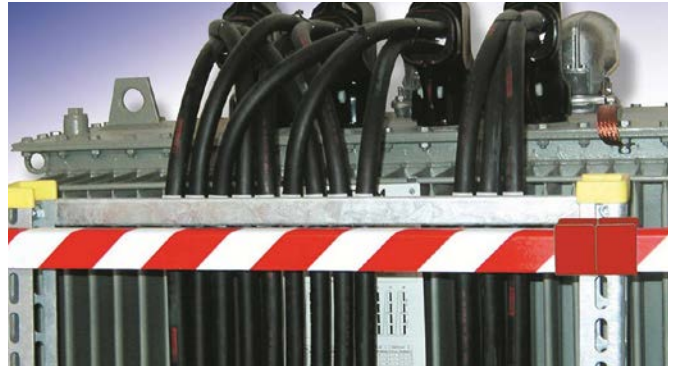
Barrier in a transformer station.
