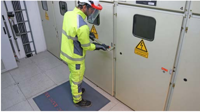
Switch room with insulating mat fitted.
