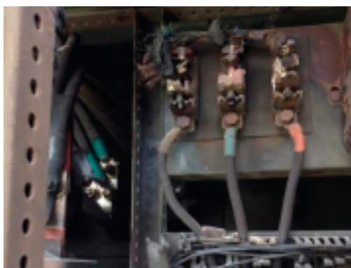
Fuses overloaded by impulse currents
